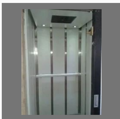
Office Passenger Lift
