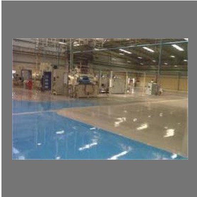
EPU Coating Services
