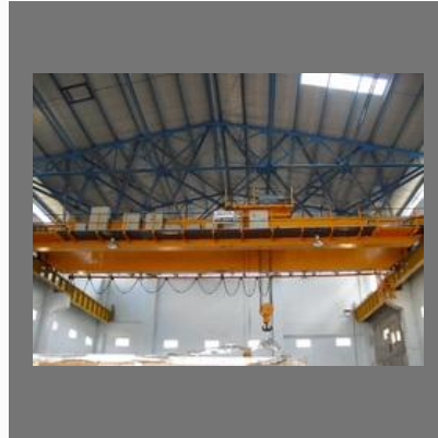
Girder EOT Crane
