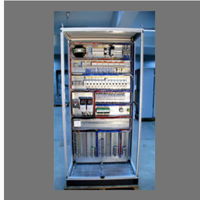
Custom Control Panels
