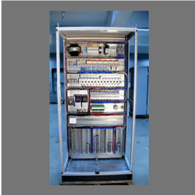
Custom Control Panels
