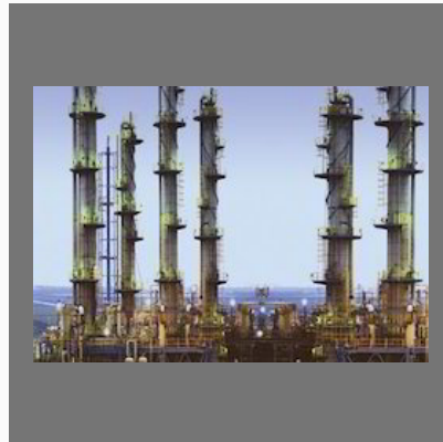
Fractional Distillation Columns
