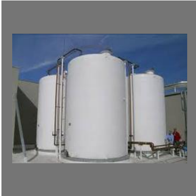
Chemical Storage Tanks
