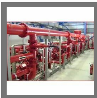
Fire safety Pipe Line
