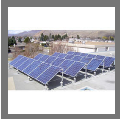
TATA Power Solar Grid Tie Rooftop Systems
