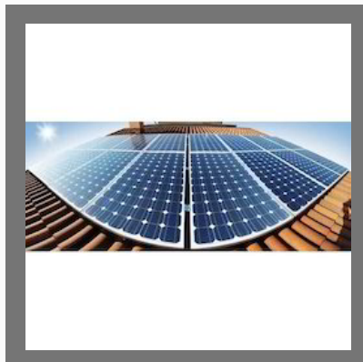
TATA Industrial Solar Rooftop System
