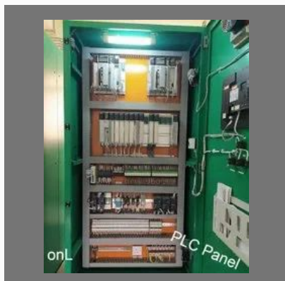
Vfd And Plc Panel
