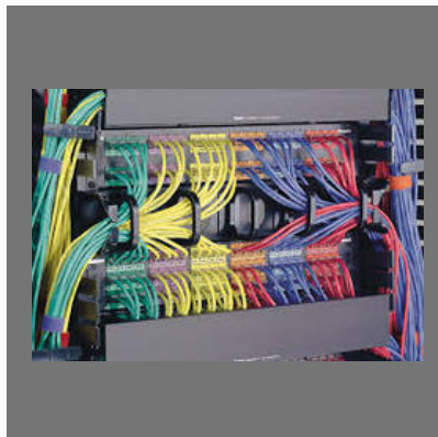
Structured Cabling Solutions
