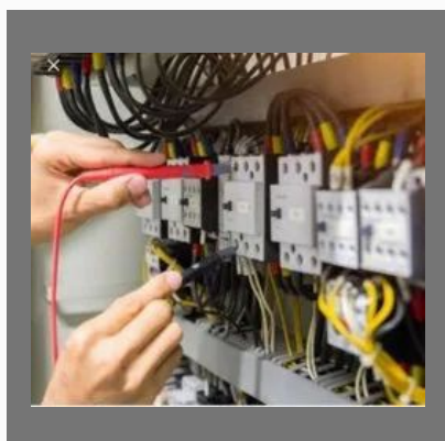
Electrical Preventive Maintenance Service
