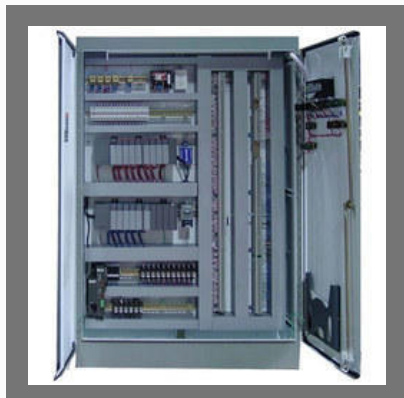
Three Phase Electric Control Panel
