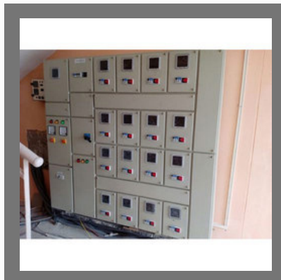
Automatic Panel Board
