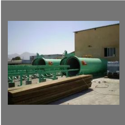
Vacuum Pressure Impregnation Plant
