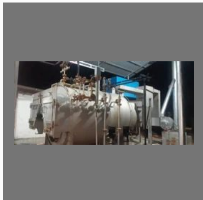
Coal Fired Steam Boilers
