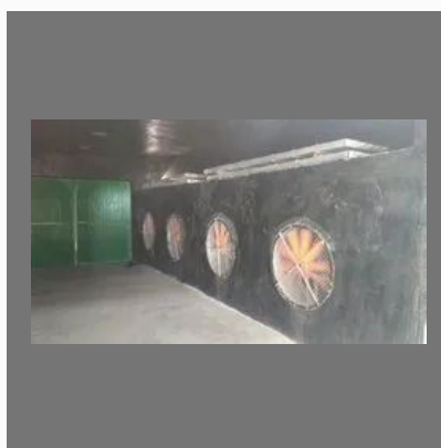
Wood Seasoning Kiln Side Wall Fan Type
