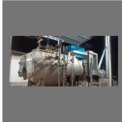
Oil Fired Steam Boiler
