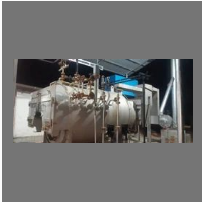
Solid Fuel Boiler
