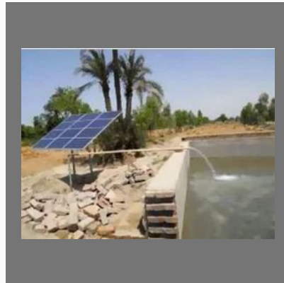
Energy Saving Solar Pumps
