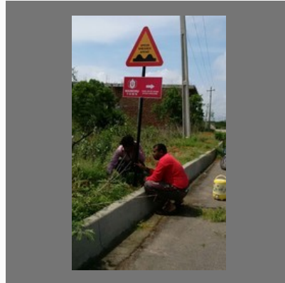
Direction Sign Board
