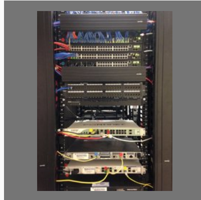
Network Infrastructure & Services
