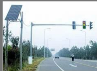
Solar Traffic Lights
