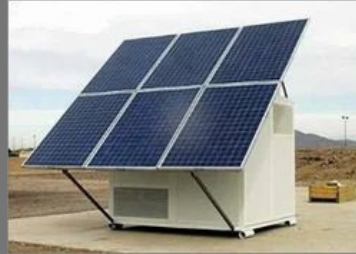
Shelter Mounting Solar Panels Structure
