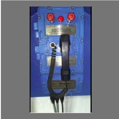
Telephone PA System
