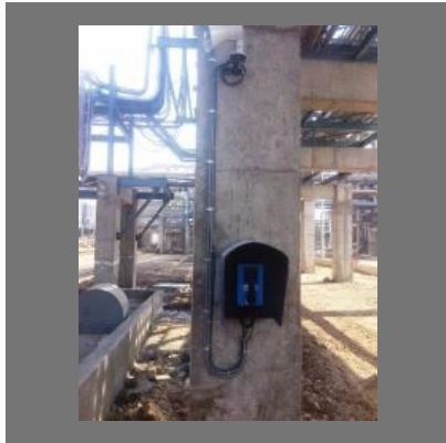
Telephone Alarm System
