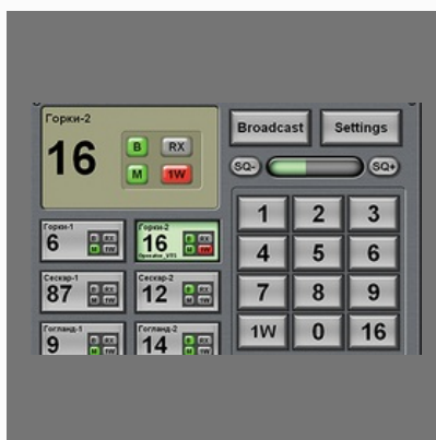
VTS Radio Water-side VHF Communication System
