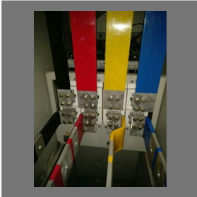
HV Power Panels
