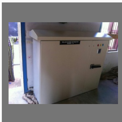
Electric Control Panel
