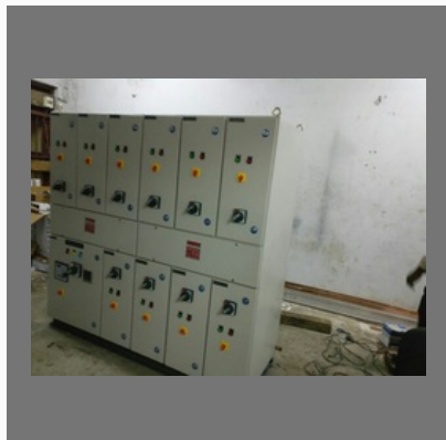
Electric Control Panel
