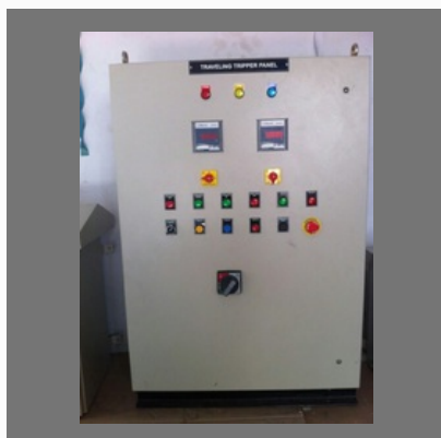
Control Panel Board
