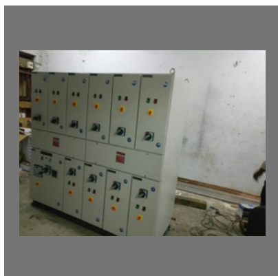
Electric Control Panel
