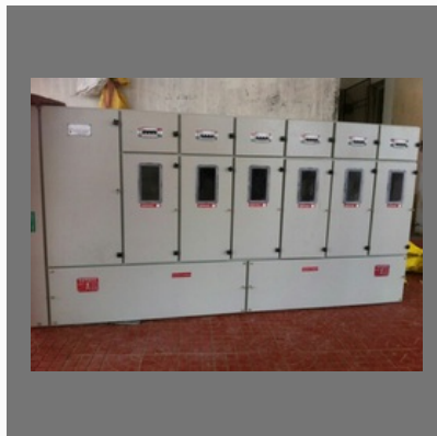
Control Panel Board
