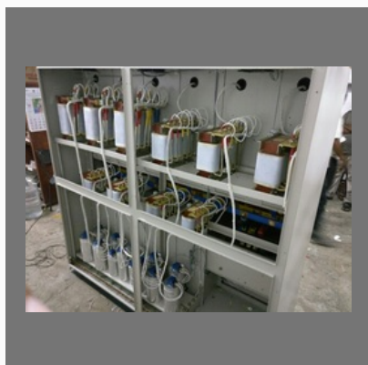
Industrial Control Panels
