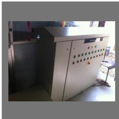
Electrical Control Panel
