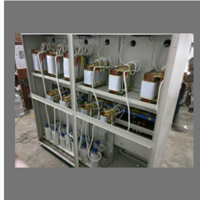
LT Distribution Panel
