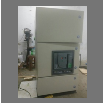
Heavy Electric Control Panel
