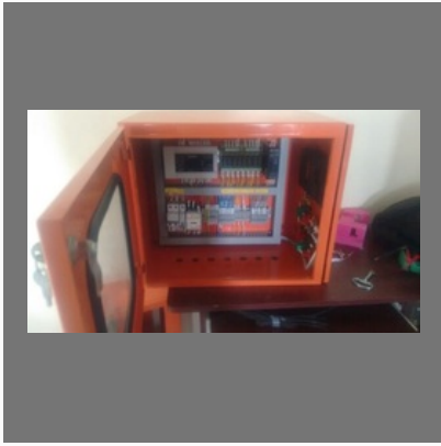
Hydropress Machine Control Panel
