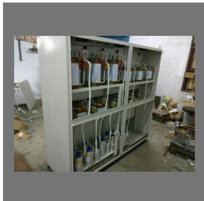
Electric Control Panel
