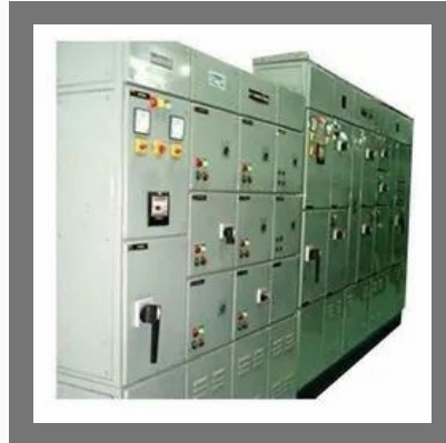
Capacitor Control Panel
