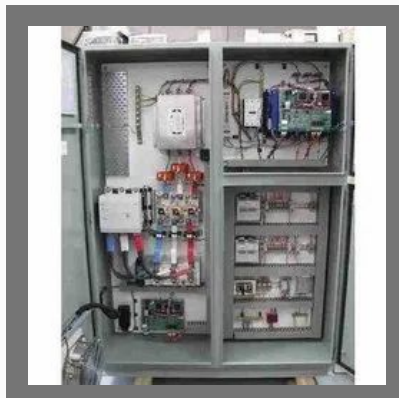
Thyristor Control Panel
