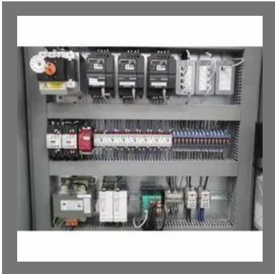
Process Breaker Panel
