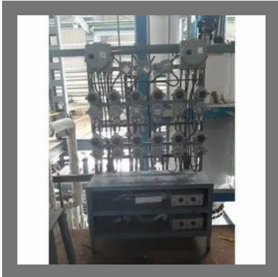
Electrical Maintenance Service
