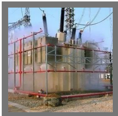
Transformer Protection High Velocity Water Spray Systems (HVWS)
