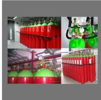
INERT (IG/541) GAS FLOODING SYSTEM
