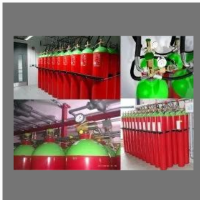
INERT (IG/100) GAS FLOODING SYSTEM
