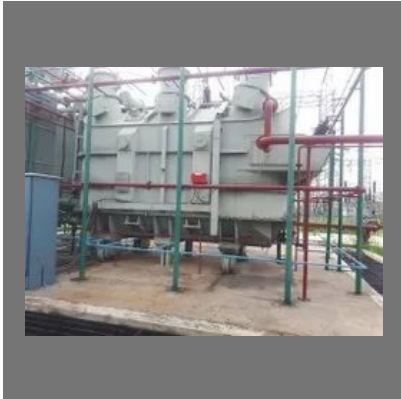
Nitrogen Injection Oil Evacuation Fire Protection System
