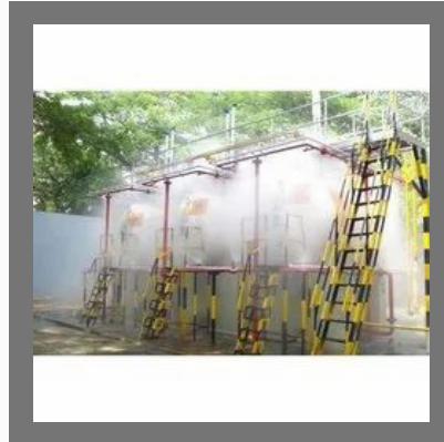
Medium Velocity Water Spray System (mvws) For Flammable Gas Storage Tanks
