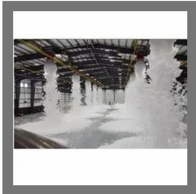
Foam Flooding System
