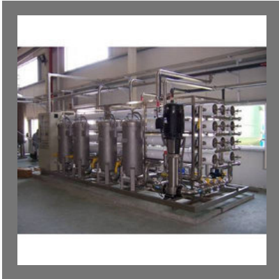
Industrial RO Plant
