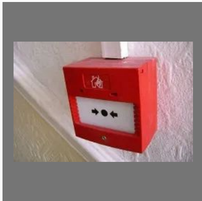
Automatic Fire Alarm System
