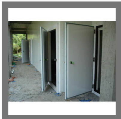
Insulated Cold Room Door
