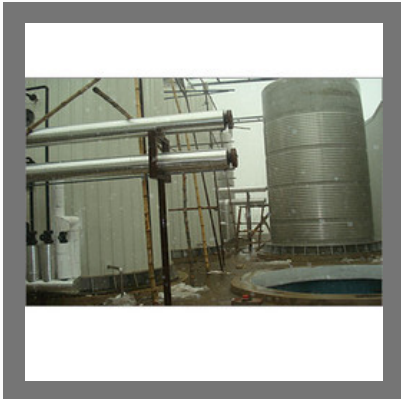
Cold Thermal Insulation Service
