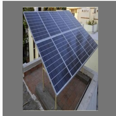
Solar Roof Top Plant
