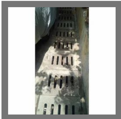
Concrete RCC Chamber Cover
