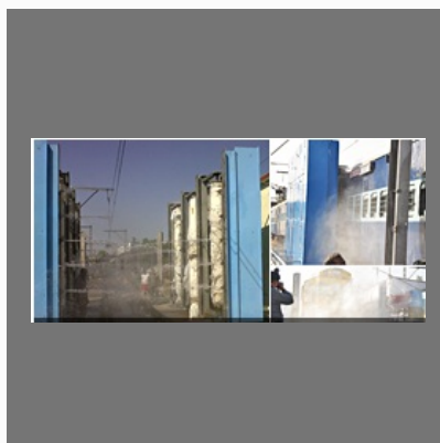
Automatic Coach Wash Plant
