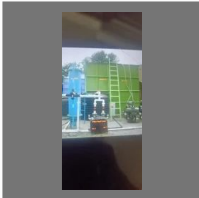
Filter Feed Pump
