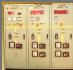
Control & Relay Panel
