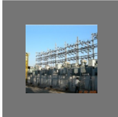
Substations & Switchyards Services
