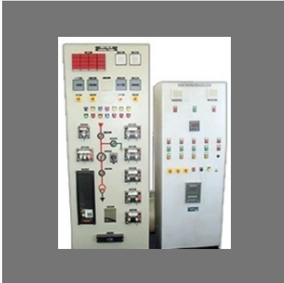
Relay Control Panel & RTCC Panel
