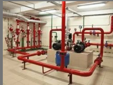
Fire Safety Service
