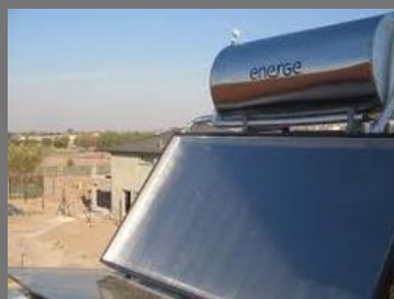
Residential Solar Water Heater
