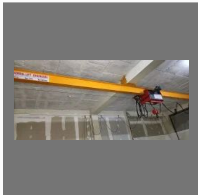
Single Girder Underslung Crane
