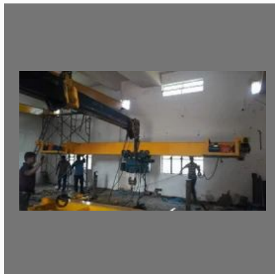
Electric Over Head Crane
