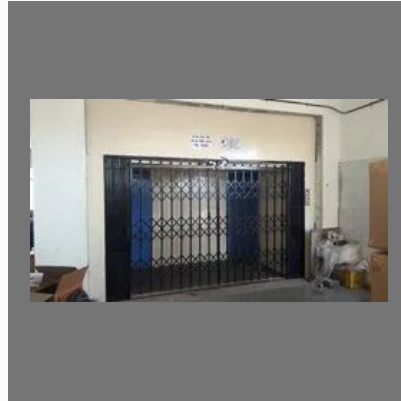
Hoist Operated Goods Lift
