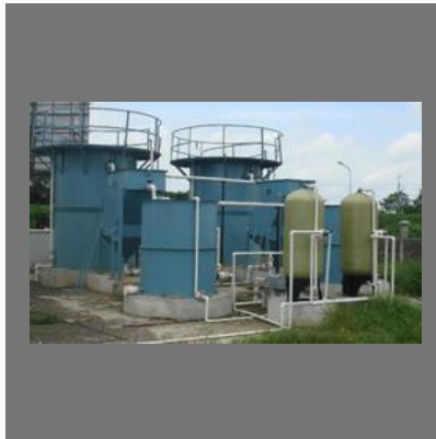
Industrial RO Plant
