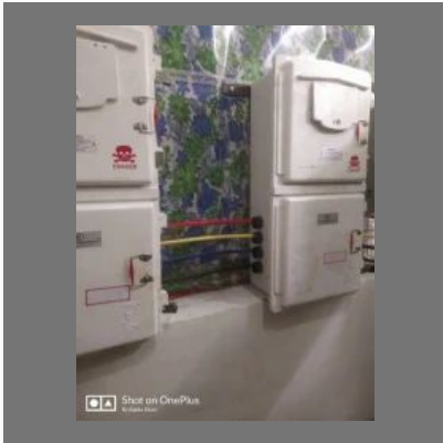
Residential Electrical Works
