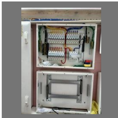
Electrical Control Panel
