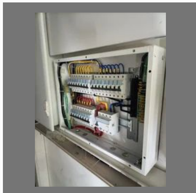
Electrical Control Panel
