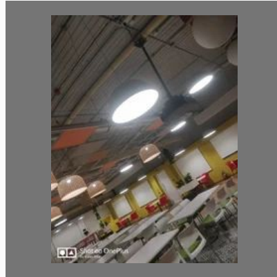
Commercial Electrical Works
