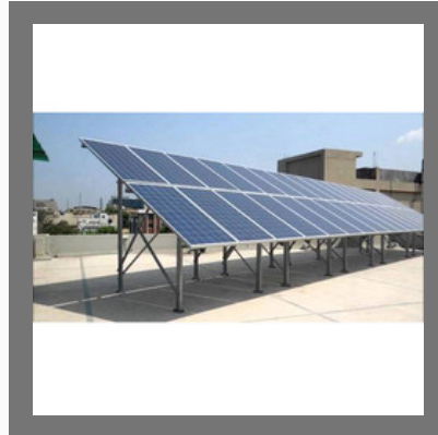
Subsidies Solar Rooftop System
