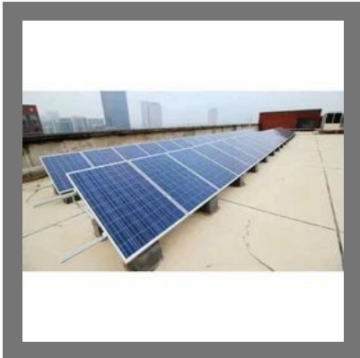
Single Phase Solar On Grid Rooftop System
