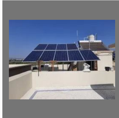
Solar Off Grid Rooftop System
