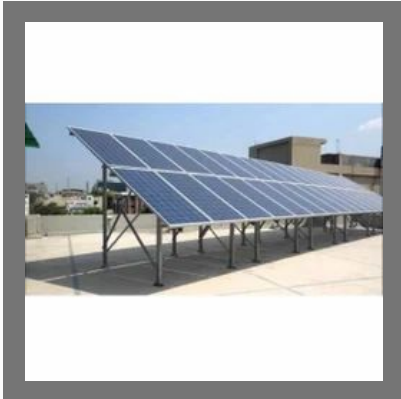
Subsidies Solar Rooftop System
