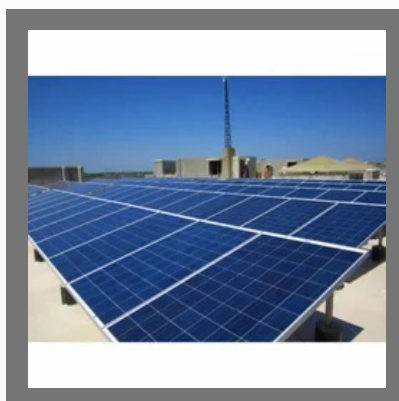
50 Kw Solar Power Plant
