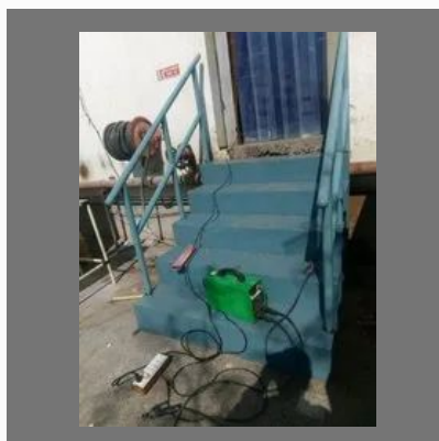
Mild Steel Staircase
