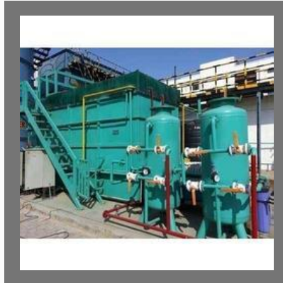
Sewage Water Treatment Plant
