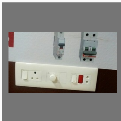
GM Legrand Electrical Switches
