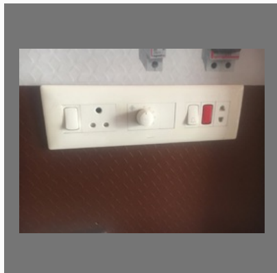
Legrand Modular Switches
