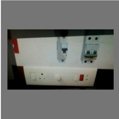
Gm Legrand Electrical Awitches
