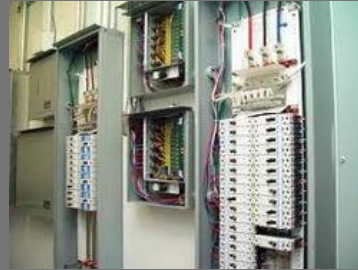
HT Electrical Installation Services
