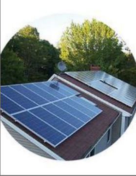
Solar Energy System
