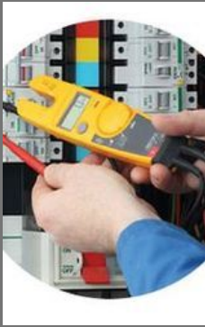
HT And LT Electrical Installations
