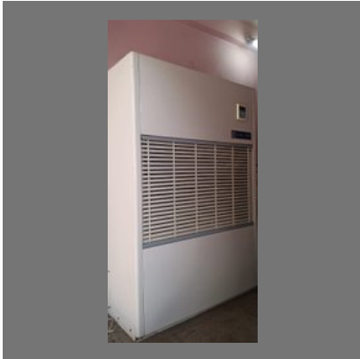
Annual Maintenance Contract For AC In Commercial Project
