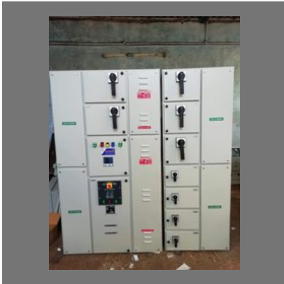
Distribution Panel With Power Factor
