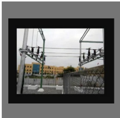
Ht Electrical Works
