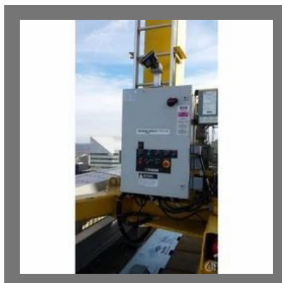
Crane Control Panel
