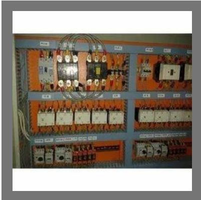
Three Phase Electric Control Panel
