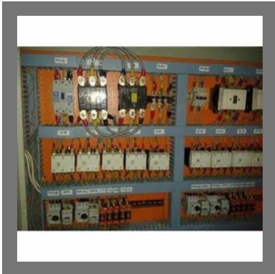
Single Phase MCC Panels
