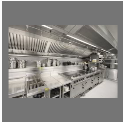
Commercial Kitchen Equipments
