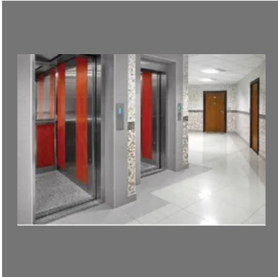
Shopping Mall Passenger Elevator
