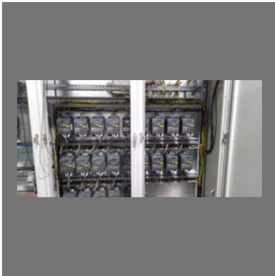
Electrical Control Panel
