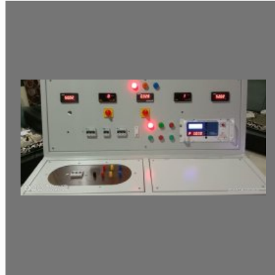
Electric Control Panel Board
