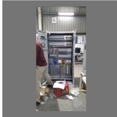
Thyristor Heater Control Panel
