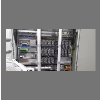
Electrical Control Panel
