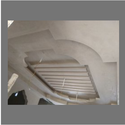
Pop False Ceiling with planks
