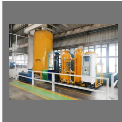
PSA Nitrogen Gas Generation Plant
