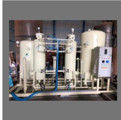
PSA Oxygen Gas Plant
