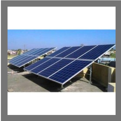
Solar Rooftop Panel
