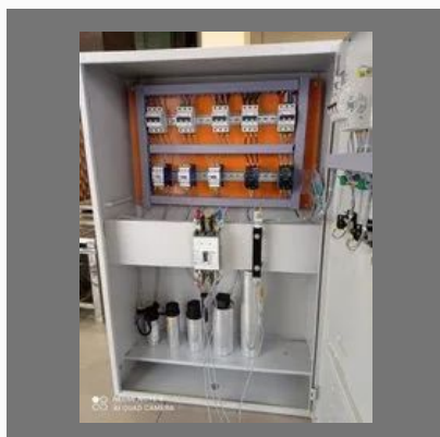
APFC Electric Control Panel
